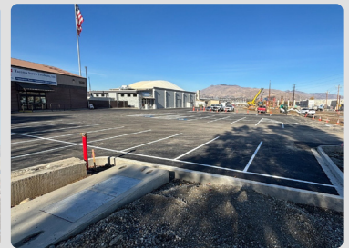
Demolition and restoration complete near the North Miller Business Park, making way for the Miller St overpass
